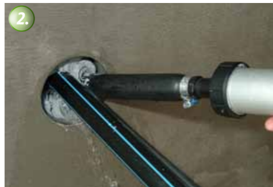
The material is pressed into place between the cable and the wall with the KÖSTER Special Caulking Gun, immediately and permanently stopping the water flow.
