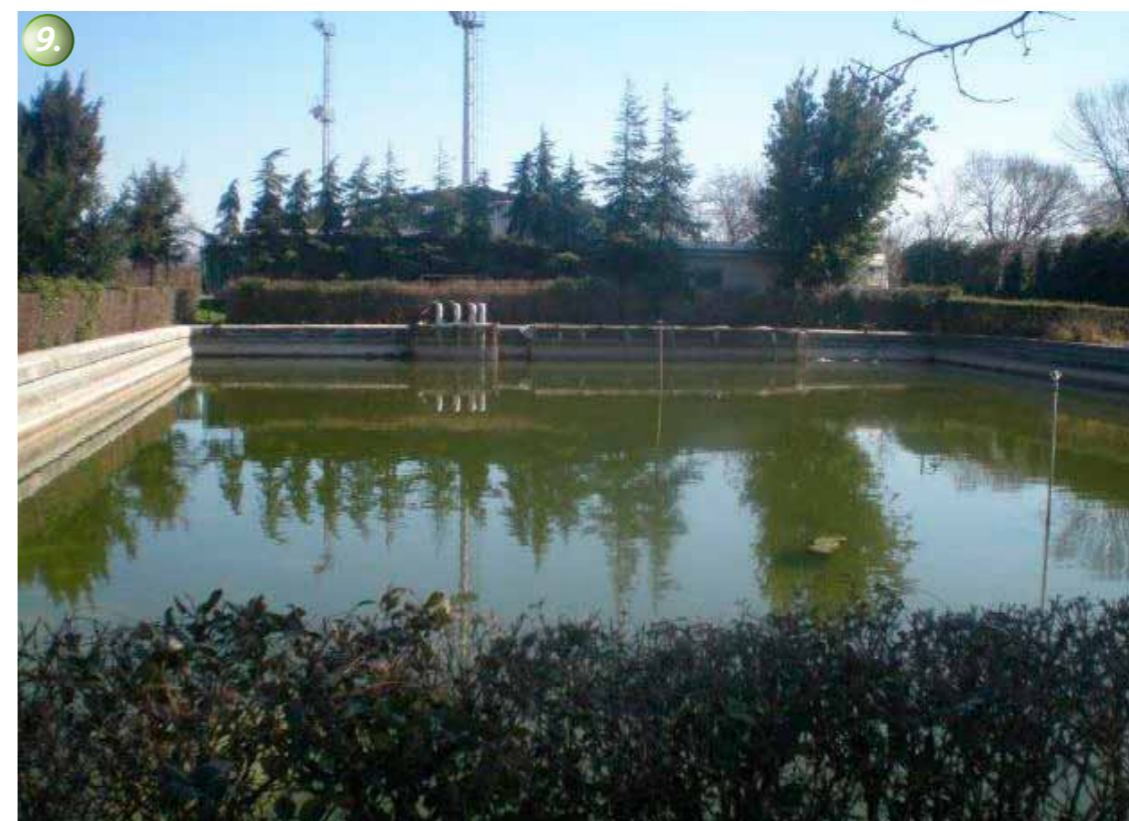
The KÖSTER joint and area waterproofing system has proved itself for years at the Veli Efendi Racetrack and still reliably serves the basin as an unfailing waterproofing.
