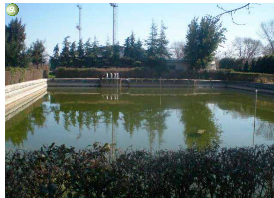
9. The KÖSTER joint and area waterproofing system has proved itself for years at the Veli Efendi Racetrack and still reliably serves the basin as an unfailing waterproofing.
