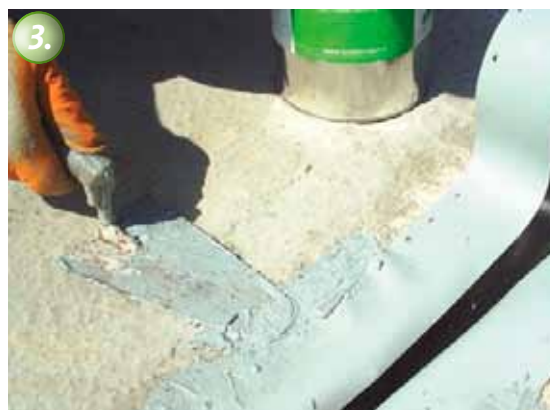
3. To give the KÖSTER Joint Tape more tolerance, it is pressed slightly into the joint.
