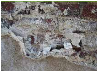
Typical damage through salt efflorescence.
