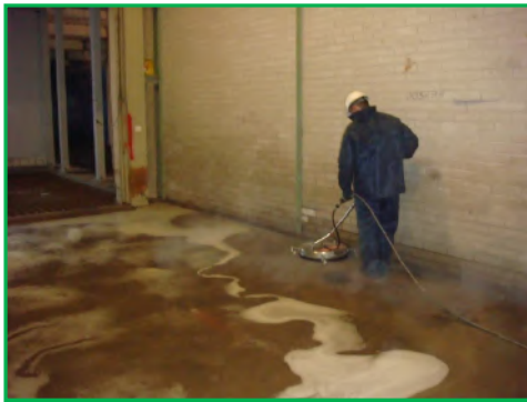
Pic. 15: Using the floor spinner to get the hot detergent / water mix with high pressure (100°C; 300bar) into the concrete to ensure removal of the oil to a sufficient depth (2-3cm)
